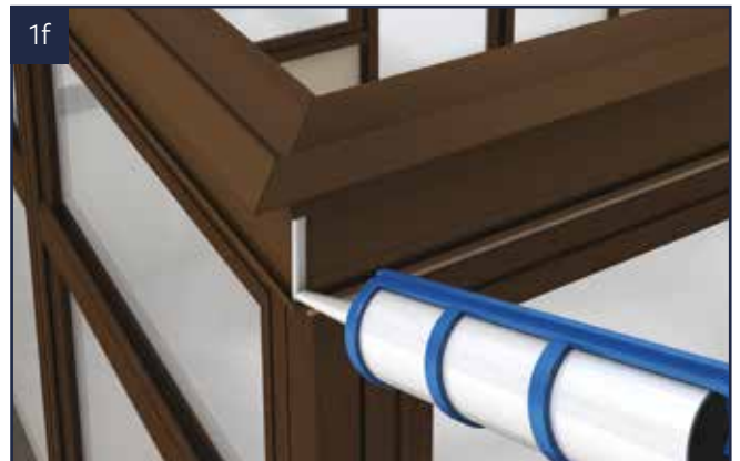
Apply a line of silicone sealant to the outer edge of the ringbeam joint.
