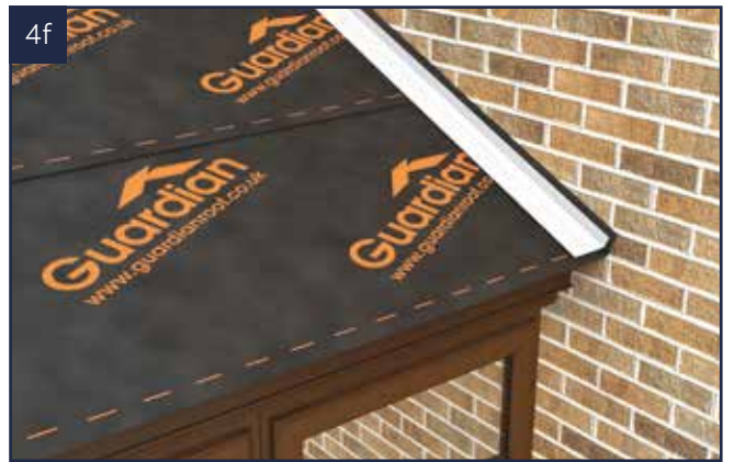
When all membrane is in place, fit the watercourse / soaker against the house wall.
