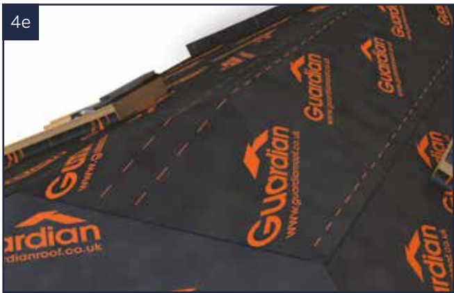
Add the final run of membrane over the apex of the roof.
