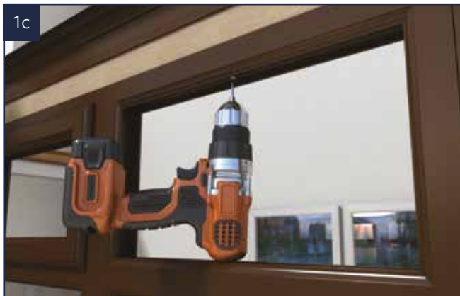
1c Remove existing glazing and fix through timber packer using fixings supplied. Fixings at no more than 150 mm from either end and no more than 500 mm centres.
