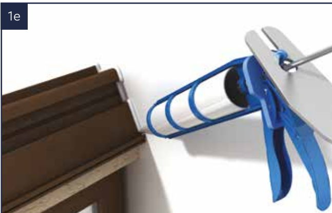
Apply a line of silicone sealant between the Ringbeam and the house wall.
