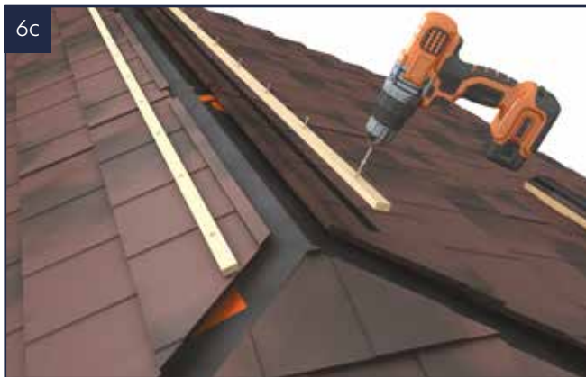
Fit timber battens and screw into place (battens must be kept dry).
