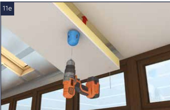
Holes for spotlights can now be cut in preparation for fitting of the lights, see appendices for light fitting.
